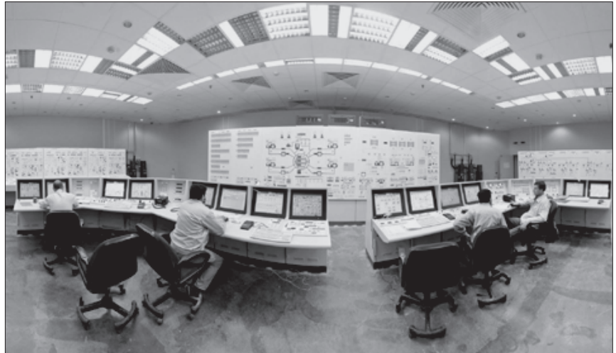
The control room at Iran's Bushehr nuclear power plant. There is no evidence that Iran ever diverted materials from a civilian to a military nuclear programme.
